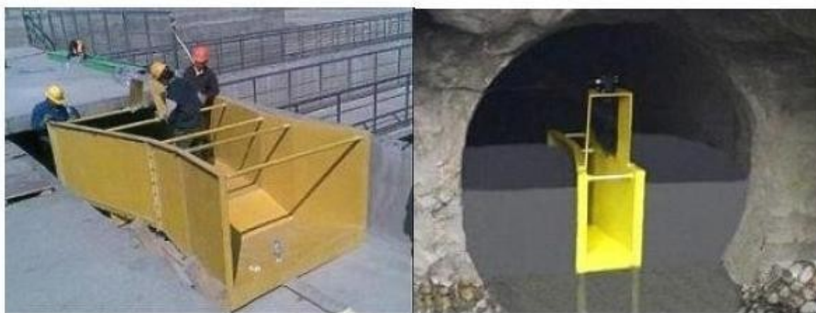
Parshall flume local installation pictures
